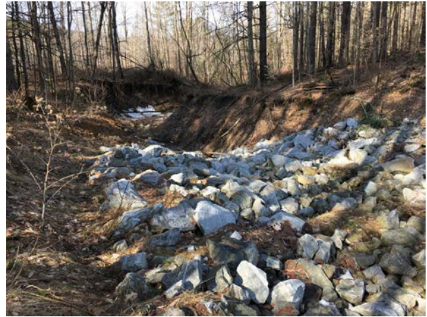
Figure 1. Significant erosion at the Pouliot Ave stormwater outfall and resultant large gully.
